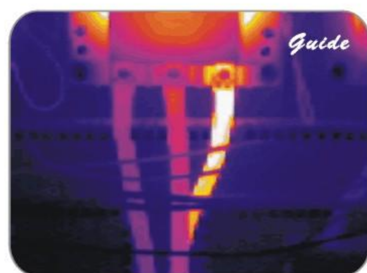
Inspect electricity hot point
